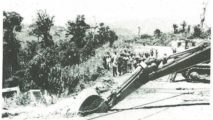
Shows tackle layout and the grader on the way up. Inquisitive onlookers in the background.
