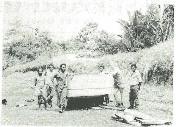
Shows SGT Dave Stewart and national helpers during repairs to towed roller at Pimaga S.H.P.
