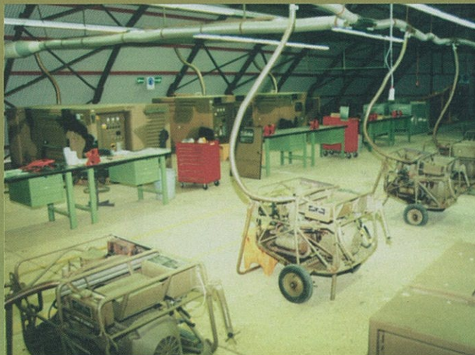
State of the art generator training facility
