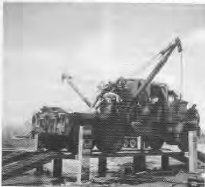
Wash point constructed by CPL Stow over a 3 day period ably assisted by CPL Pete Chalker, CFN Ford and CFN Gonninan. The Mack Wrecker was used to test load the ramps.
