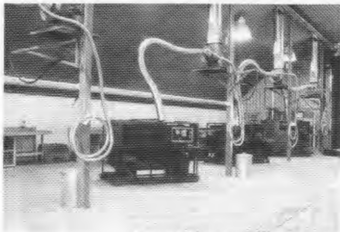
Interior of new generator training facility.
